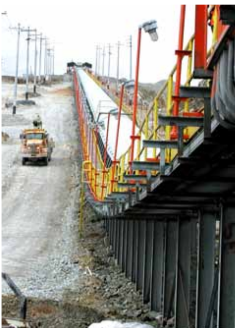
PT Freeport C201 Conveyor Installed in 1998
